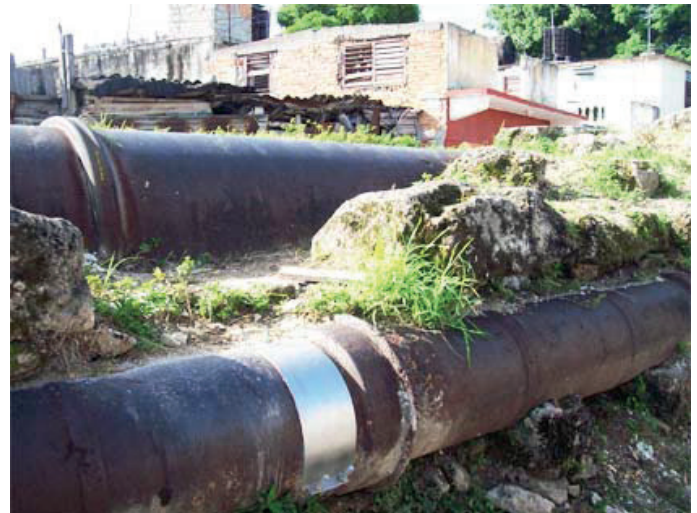
Fig. 4. Top to bottom: the iron pipes of Albear (1893) and Fernando VII (1835) showing a repair. The pipes are on top of a wall built to protect them in the street named Resguardo (protection) in Cerro municipality.
