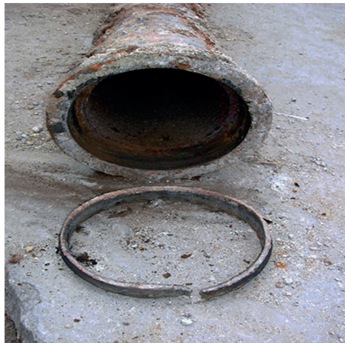
Fig. 2. In Philadelphia the joints of the pipes were filled with lead, technique that was also used in Havana.
