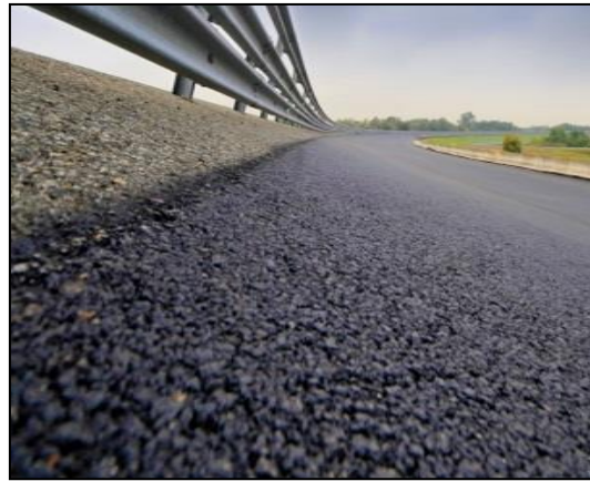
Figure 5: Segregation due to defective materials.
