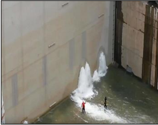
Figure 4: Dam design failure. materials.
