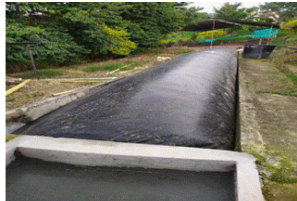
FIGURE 1. Biodigester installed at Santa Bárbara Farm.
