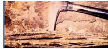
FIGURE 6. Exfoliation corrosion in a water treatment plant.
